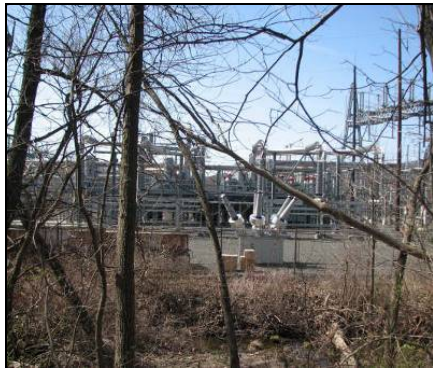
Sub-Station Power Facility
